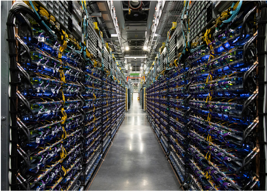
Figure 7: A TPU v4 Pod contains 4,096 TPU v4 chips and delivers more than 1 exaflop / second of computing power. This TPU v4 Pod is in a datacenter that is operating at or near 90% carbon-free energy.
